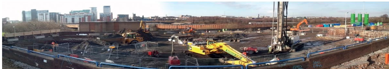
Pictures Courtesy of WSP and National Grid
